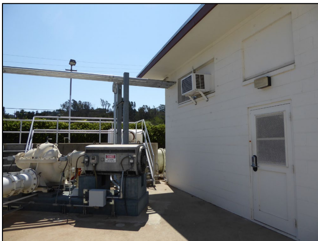
Avenue 2 Pump Plant Electrical Building
