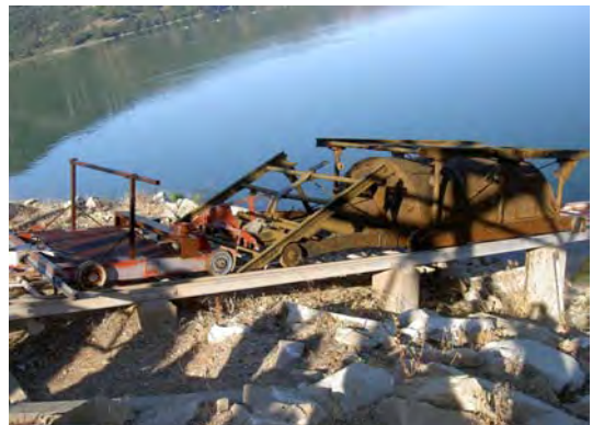
Lake Casitas' Intake Structures would be vulnerable to mollusk.
