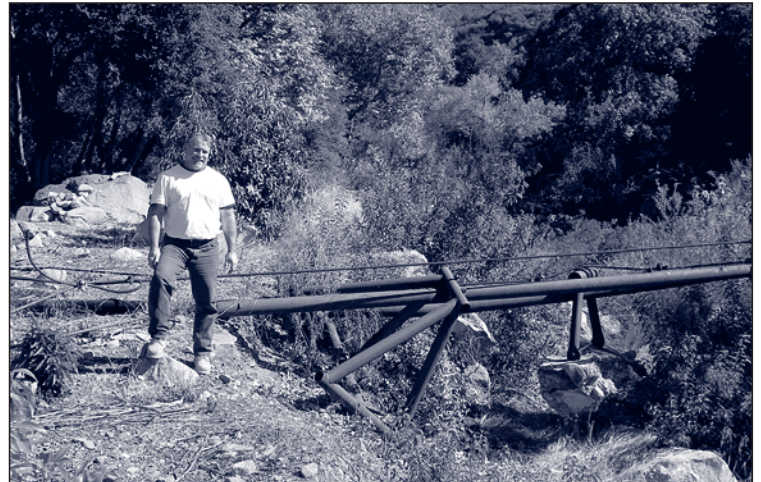
Larry Catlett, general manager of Senior Canyon Mutual Water Company, stands next to a main distribution line which is slated for replacement with grant funds. This line is almost completely filled with mineral deposits.
